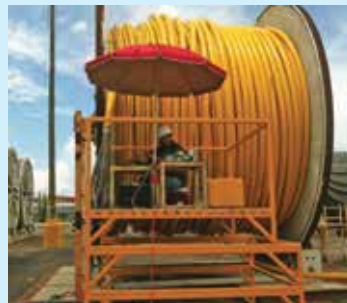
When terminating the fiber optics within a complex cable, a breakage of an optical fiber can cause the complete retermination of all the elements within the cable. This can cause a delay of several days.
